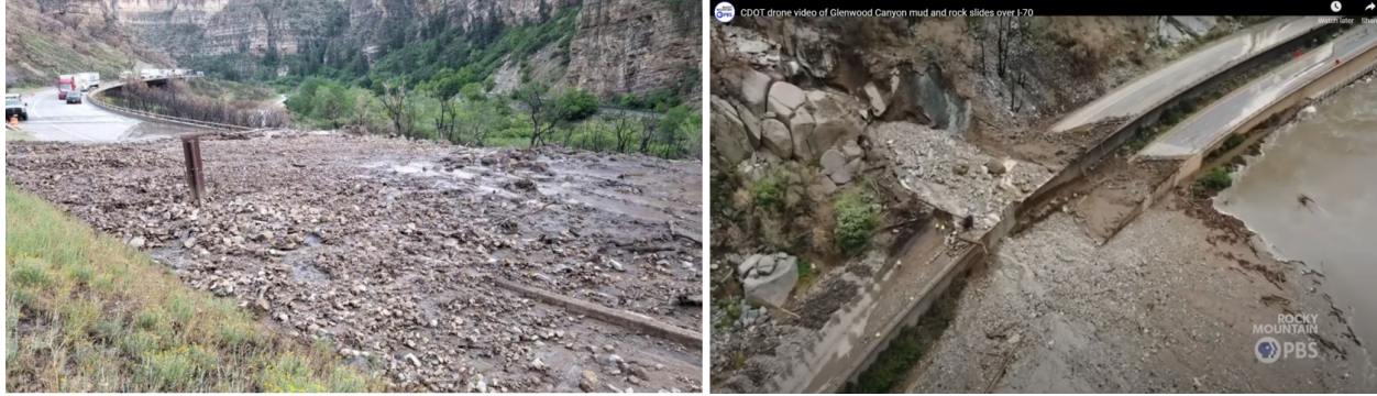
Figure 38: Images of the damage from debris flow that occurred in Glenwood Canyon on July 22, 2021 due to rain falling on over the Grizzly Creek Fire; courtesy of (left) Meckles and Bianchi (2021) and (right) still taken from drone footage in Stroud, J. (2021).
