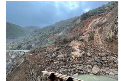
Landslide on Hwy 1 near Mill Creek in Monterey County ( Caltrans )
